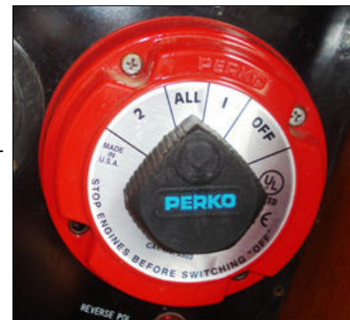
Here's the typical main battery switch. Note the warning (Stop engines before switching off)
